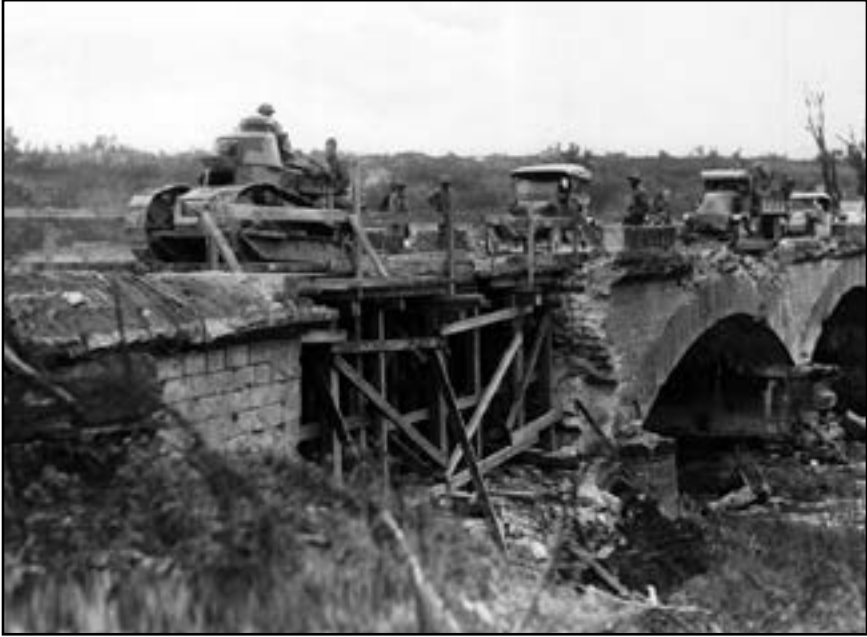
Figure 3.2. Renault FT tanks and other military vehicles cross a stone bridge repaired by Companies A and E, 103rd Engineers, 28th Division, near Beureuilles, Meuse, 28 September 1918. Courtesy of the US Army Engineer School.
