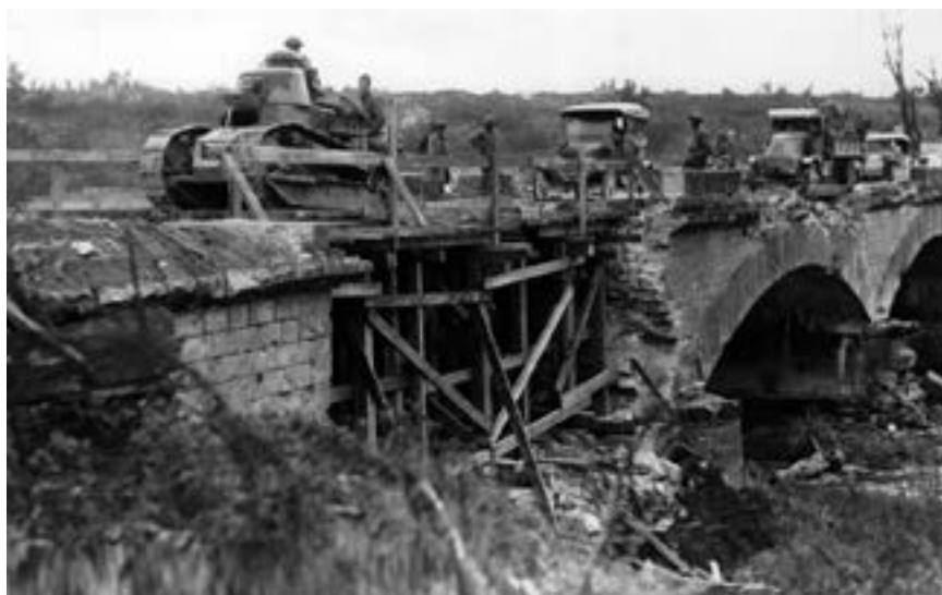
Figure 2.1. Renault FT tank and other military vehicles cross a stone bridge repaired by 203rd Engineer Regiment at Boureuilles, Meuse, 28 September 1918. Photo courtesy of the US Army Engineer School History Office.
