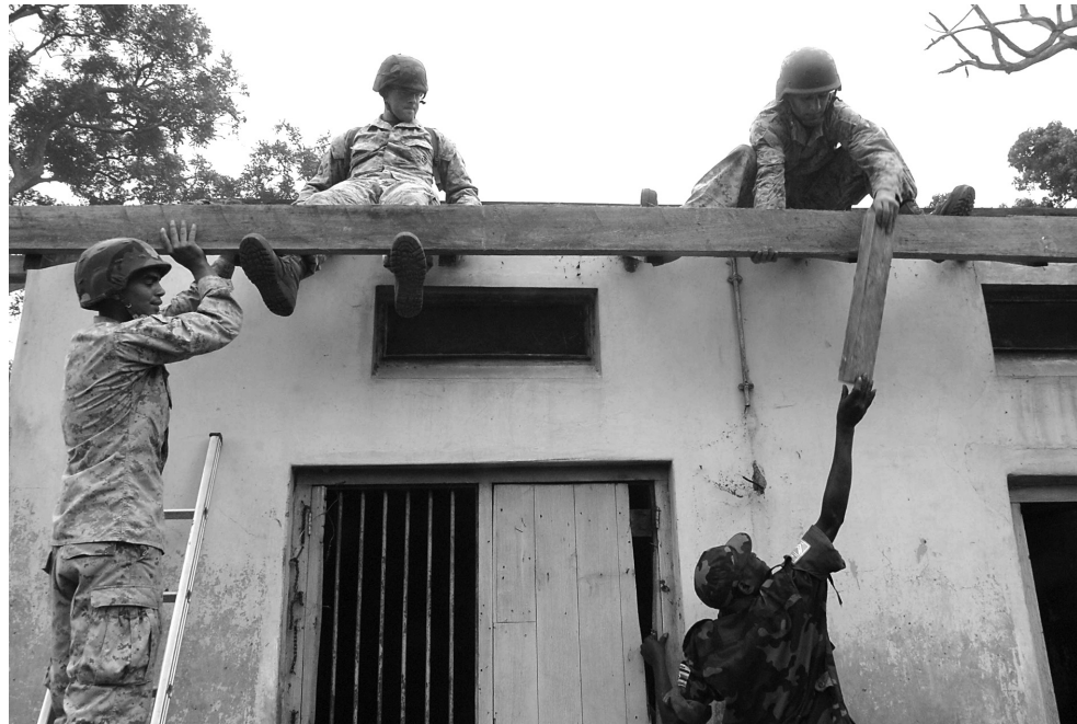
Marines assigned to Bridge Co. “A,” 6th Engineering Battalion, and soldiers of the Ugandan Peoples’ Defense Force work together to build a new roof for a nurses’ cottage during a Medical Civil Action Project (MEDCAP) in Serere, Uganda, as part of Exercise Natural Fire 2006, 20 August 2006.
