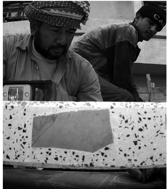
Iraqi workers hired to build steps beside the Research Triangle Institute Center in Dhi Qar Province, An Nasiriyah, Iraq, 10 January 2004.
