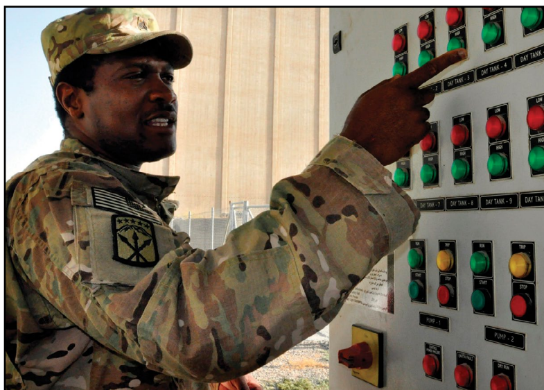
(Photo by Jasmine Chopra-Delgado, U.S. Army Corps of Engineers) Sgt. Koutodjo Ayivi, a prime power production specialist and contracting officer's technical representative with the U.S. Army Corps of Engineers' 249th Engineer Battalion, points to electrical equipment 10 August 2013 at the Bagh-E Pol power plant in Kandahar, Afghanistan. The Army faces stiff competition from colleges, other military services, and civilian employers for recruits with the potential to learn complex skills like those of Ayivi.
