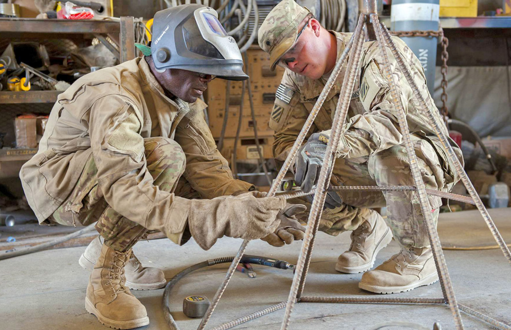
Sgt. Patrick Lewis, left, levels a piece of rebar that will reinforce a culvert denial system, with the help of Spc. Jonathan Carpenter on June 11, 2013. They are both in B Company, 703rd Brigade Support Battalion, 4th Infantry Brigade Combat Team, 3rd Infantry Division, at Forward Operating Base Shank, Afghanistan. (Photo by Sgt. Julieanne Morse)
